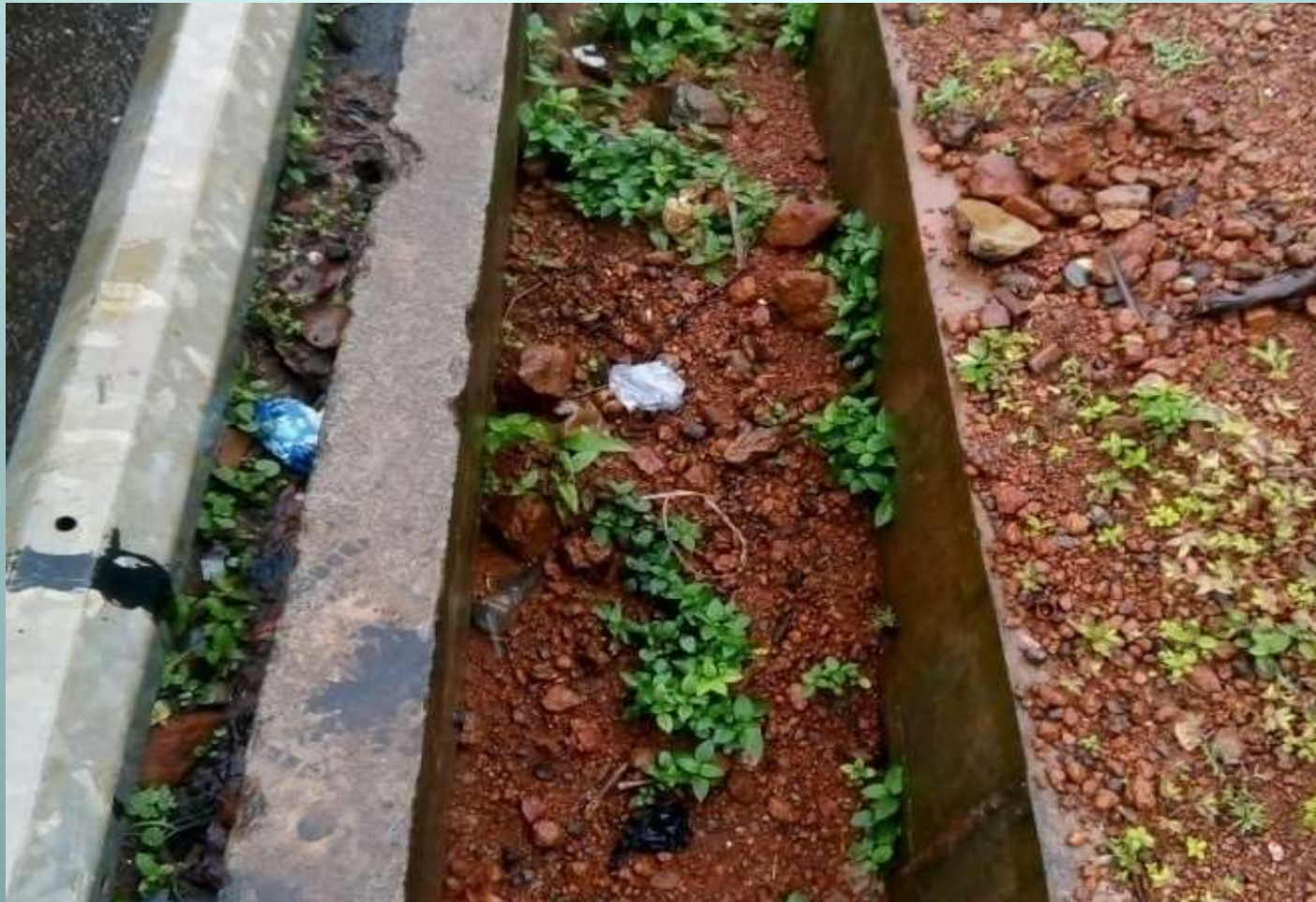
Siltation in road gutters
