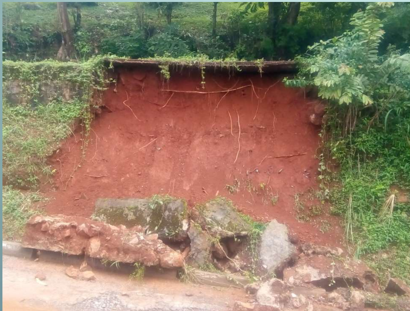
Shallow slip Failure – FBC Mount Aureol, 2019
